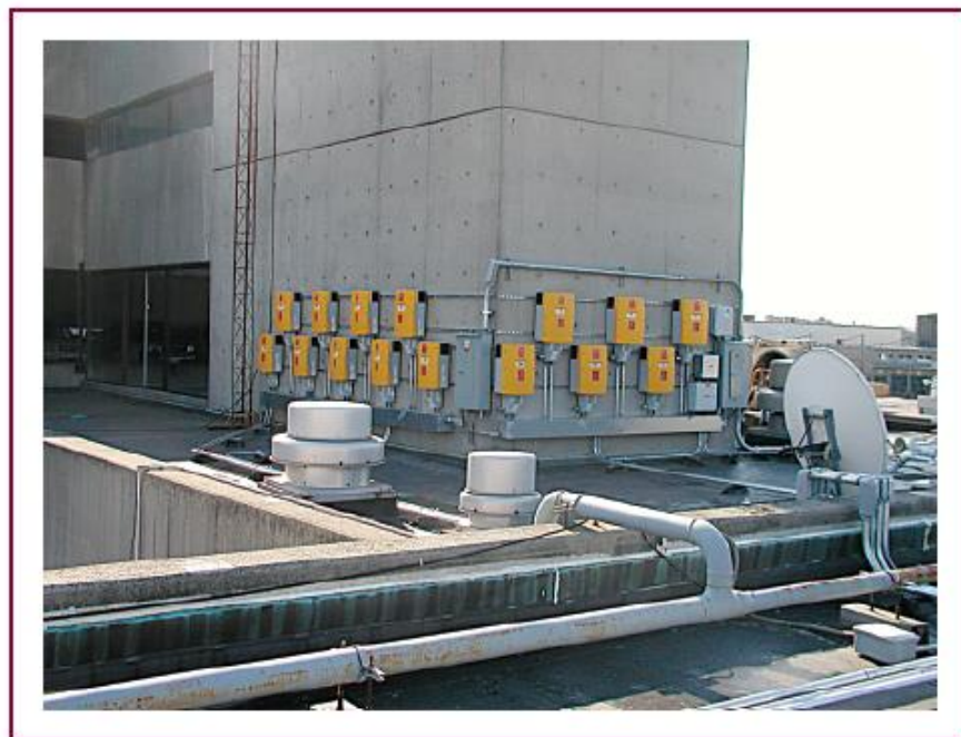
EXHIBIT 690.10 Rooftop utility interactive inverters. (Courtesy of Solar Design Associates, LLC)
