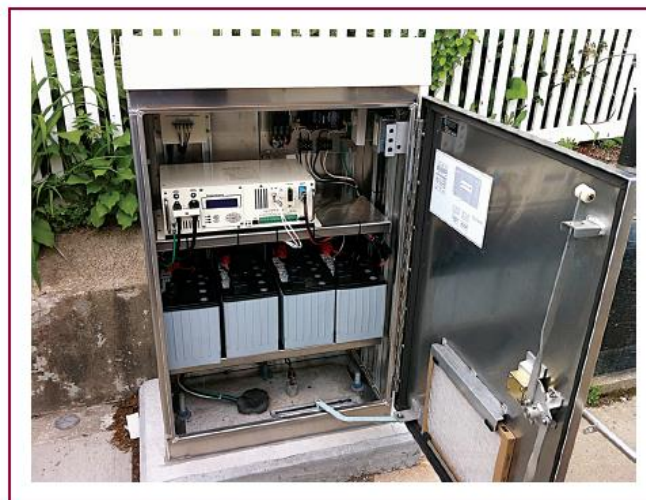
EXHIBIT 690.4 Stand-alone system components. (Courtesy of Solar Design Associates, LLC)
